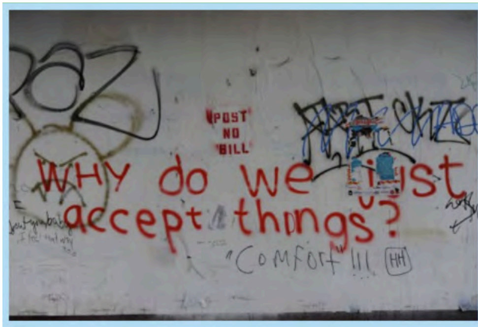
Figure 6. Kilgore community bridge tagging
